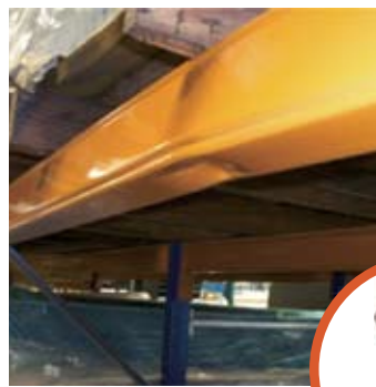
Damaged beams should be replaced.
